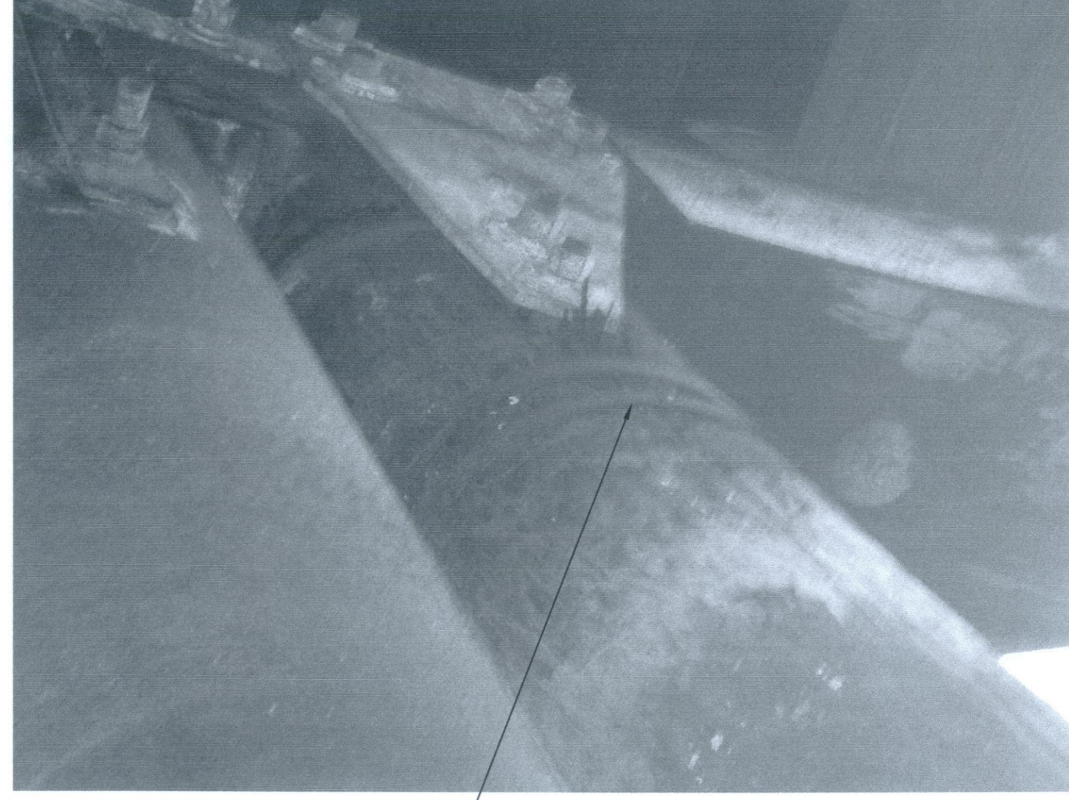
BROKEN REPAIR BANDS
