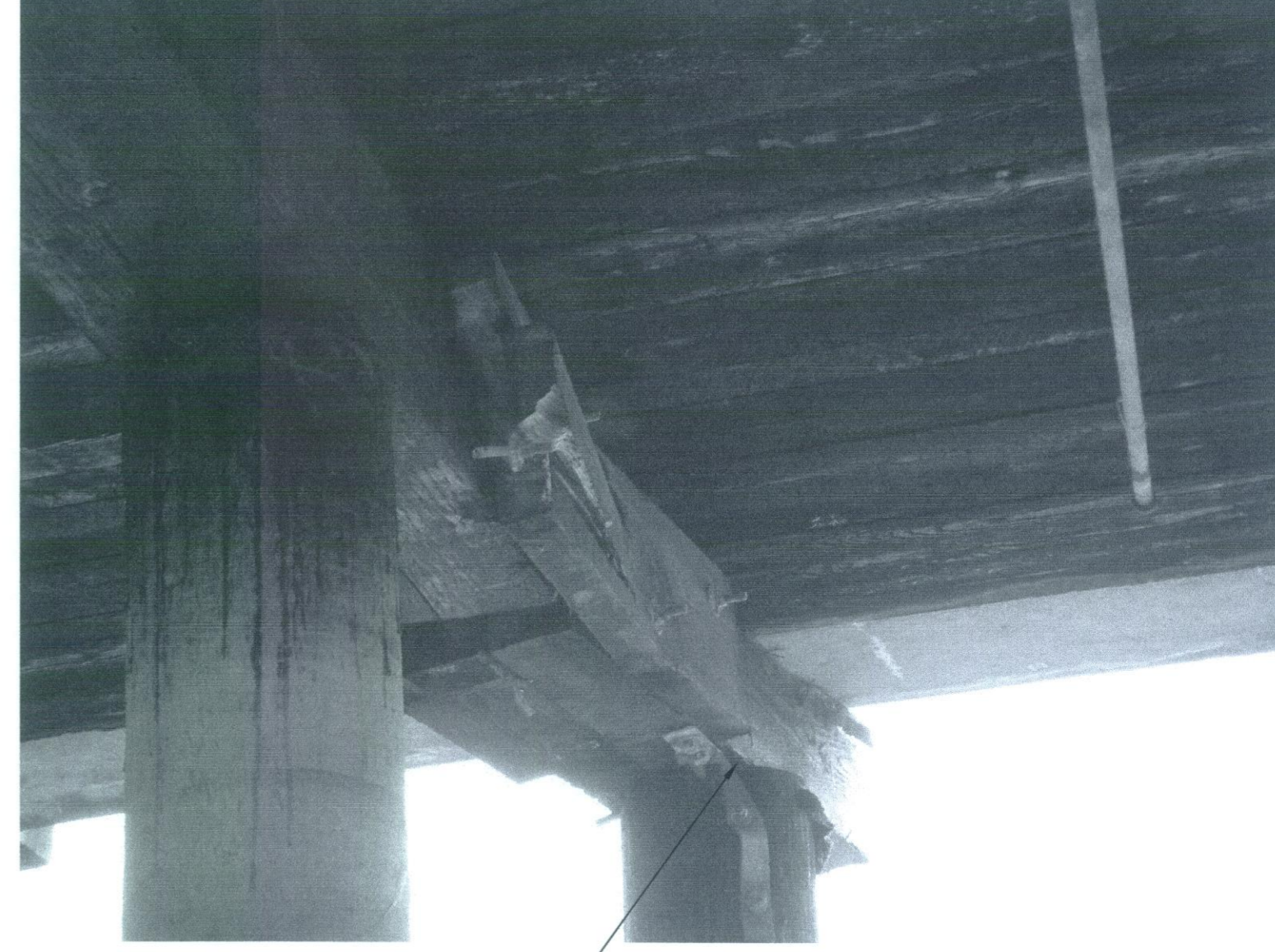
BROKEN PILE CAP SPLICE
