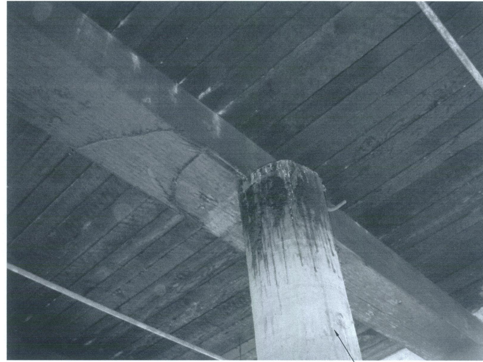
PILE BEARING LOSS
